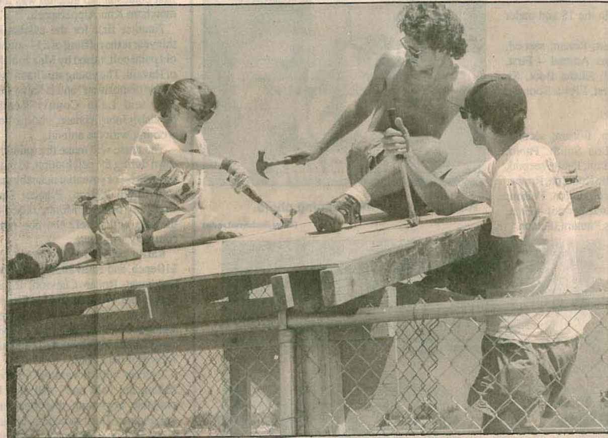
New dugout at the Ronan city ballfields takes shape under the hammers of Visions International members Beth Geller of Deerfield, Ill.,
